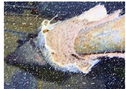
Fig.9 – Pipe insulation containing asbestos
